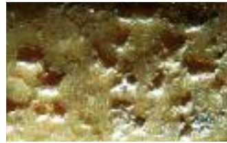
Erosion damage due to shafts that are too smooth
